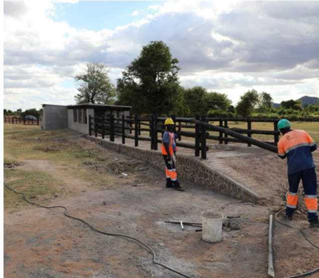
Rehabilitation of Agoni Dip Tank The company reconstructed Agoni Dip tank in Tandirwa Village, Chiadzwa, to enable the community to have an effective dip tank facility so their livestock is not subjected to tick-borne diseases and other related diseases
