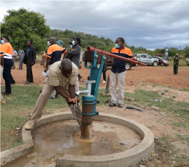
Borehole repairs The company rehabilitated 12 boreholes in Ward 29 and 10 in Ward 30 in the Chiadzwa area to afford the community access to unpolluted water.
